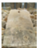
Every stone tile was taken off the roof, cleaned and put back with a new peg to hold it.
